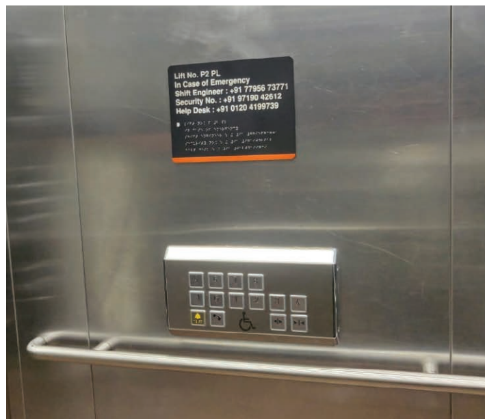
Figure 22 Lift with horizontal control panel, railings and emergency information in accessible format
